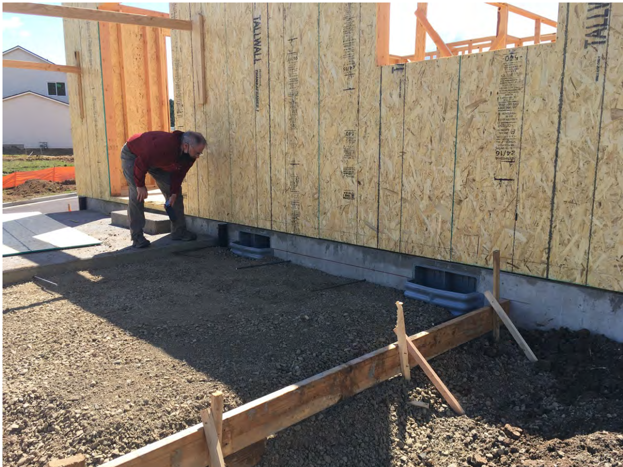
Steve looking for cracks (what else?) in the foundation of their new house.
