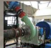
Test set up centrifugal pump
