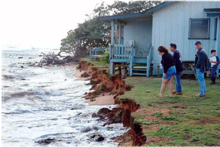
Erosion at Aliomanu Bay, Kaua'i - Coastal erosion is a significant emotional and financial burden on homeowners. ~Photo by Dennis Fujimoto of Garden Island News
