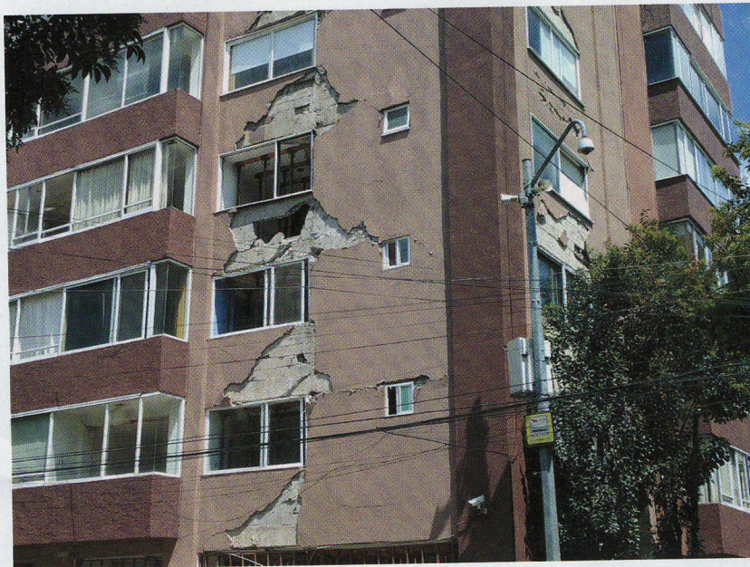
This apartment building in Mexico City was damaged during the M7.1 Puebla earthquake on 19 September 2017. One of the 12,000 pole-mounted sirens used to issue SASMEX warnings is visible in front of the building. Credit: Elizabeth Cochran
