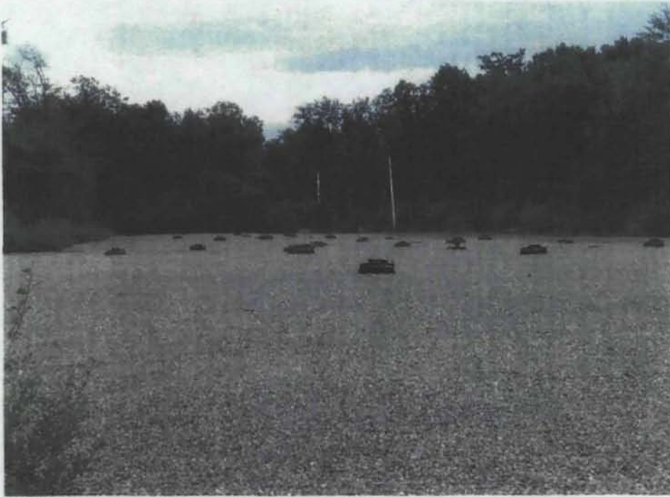
AS/SVE System Layout (looking south).
