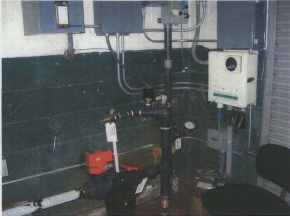
Photograph 1. Influent Piping (recently replaced)
