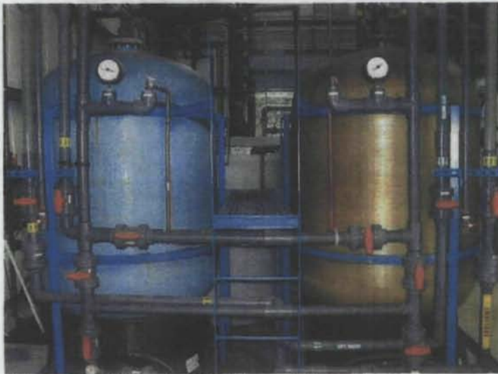
Water GAC Vessels (800#/vessel) in series.
