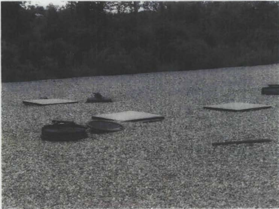
Center of AS/SVE System where SVE is divided.
