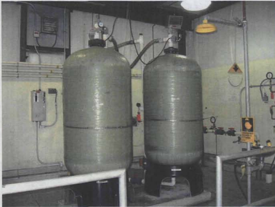
Photograph 1. Granular Activated Carbon Units (GES reported a leak at valve at top of unit on the right)
