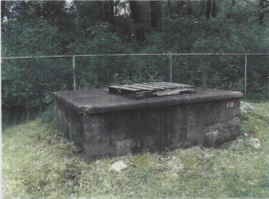
Riley Well Enclosure.
