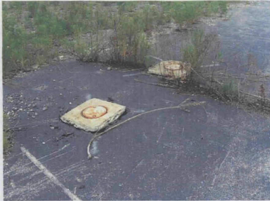
Photograph 3. Monitoring Wells G16S and G16D (Note that the concrete pads and valve boxes are dislodged from the pavement)
